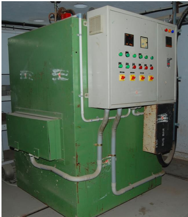
Fig.7 Steam Boiler and Controls
