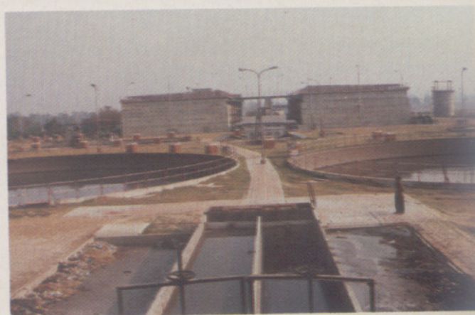
Fig 75. 36 MLD tannery waste water UASB treatment plant at Jajmau, Kanpur
