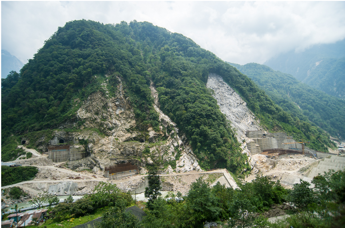
Figure 2: Construction of the Teesta III project at Chungthang on the edge of Khangchendzonga National Park proceeding without SC-NBWL clearances. Note the extensive forest cover and large landslides at the construction site.
