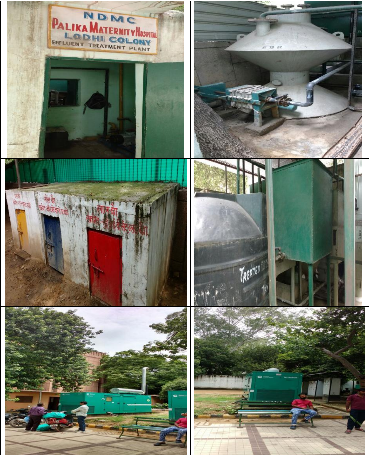
Pictures indicate ETP and DG sets in Palika Maternity Hospital
