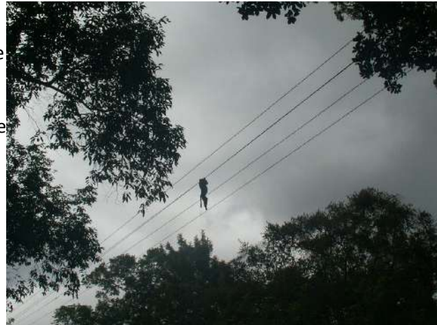
A lion-tailed macaque electrocuted while trying to use a powerline to cross a canopy gap across a road through a rainforest fragment in the Anamalai hills (Photo: M. Ananda Kumar)
