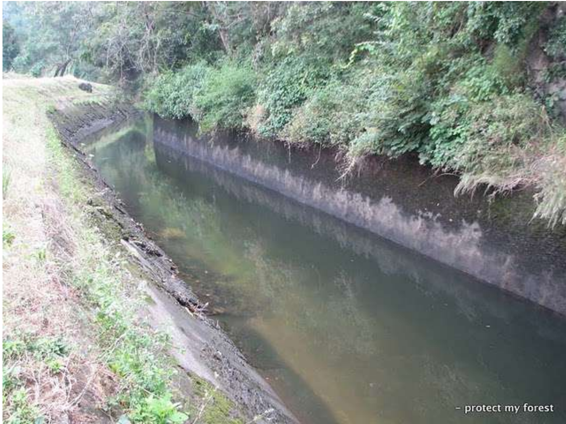
Photograph showing steep sides of Contour Canal that poses hazards to wildlife
