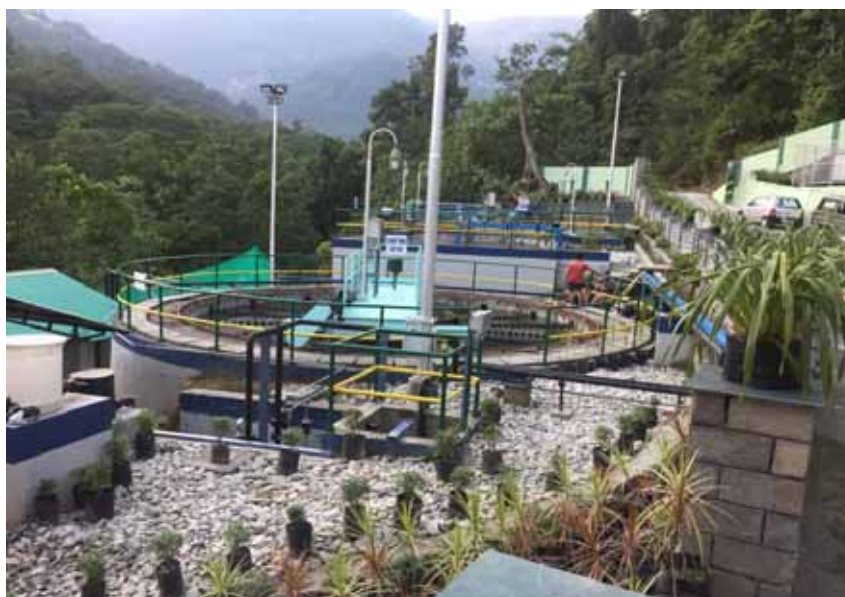
3.5 mld Sewage Treatment Plant at Zone-IV (Gangtok) constructed under NRCP
