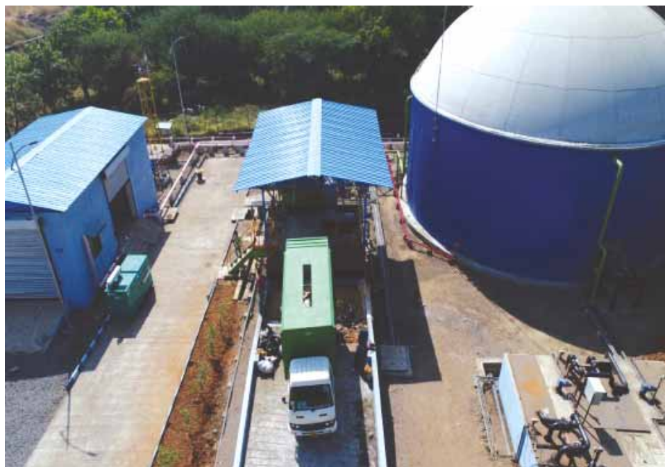
Waste to Energy (Bio-methanation) Plant commissioned at Nasik, Maharashtra on November 29, 2017
